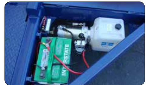
Full contained power compartment
